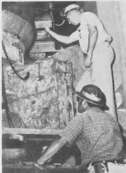
CHECKING THE installation of new skirt plates are R. C. Bergfield and Nasario Tromp.
